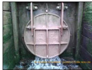
Figure 3: Modern one-way tide gate or aboiteau structure along the Grand Pre dyke in the Cornwallis Estuary.
